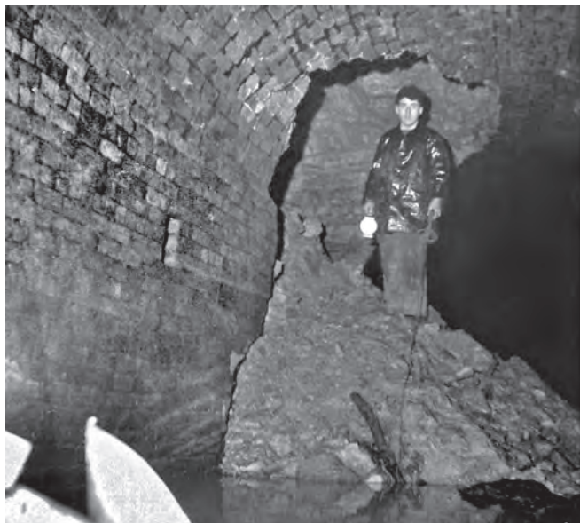
A collapse of the side wall ¾ mile from the California portal in 1961. Photo from Edwin Fasham, Lapal Canal Trust
